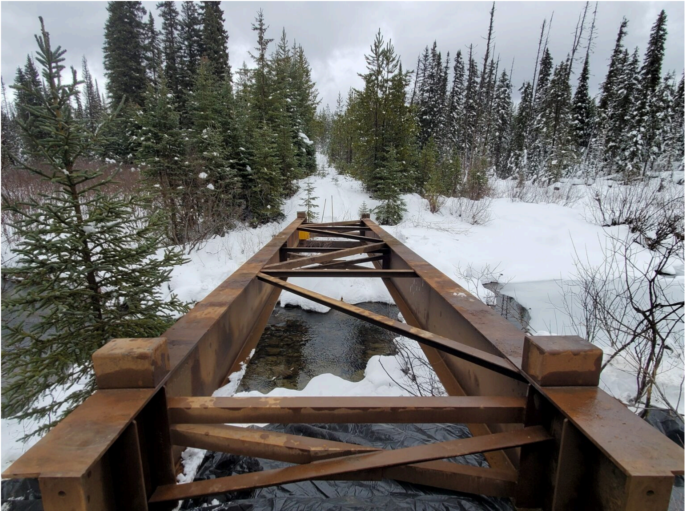
Image 2: Temporary Bridge Installation to Access Tailings Study Area (CNW Group/Defense Metals Corp.)
