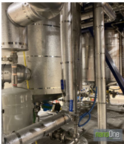
Figure 1. Two new reactors with capacity of 200 tpa
