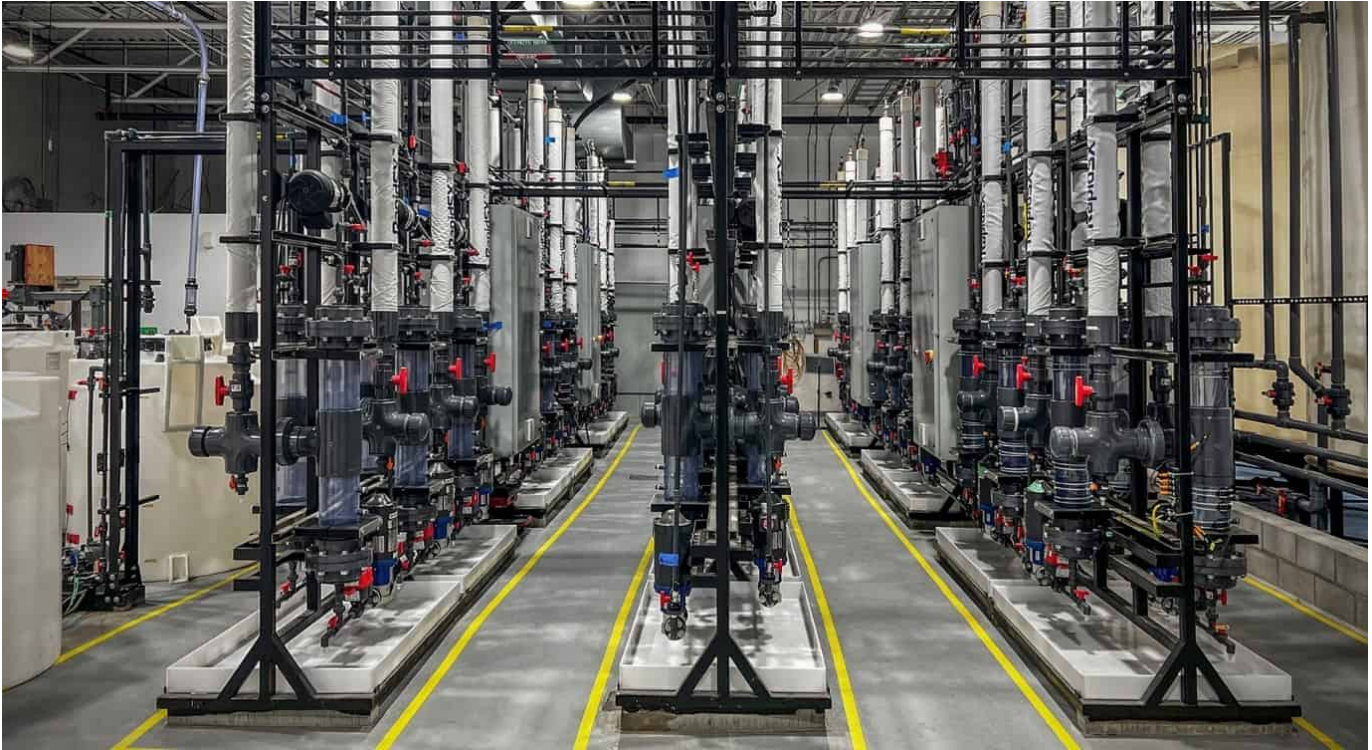
Figure 2 – The RapidSX™ Technology Platform Demonstration Plant in Kingston, Ontario, Canada
