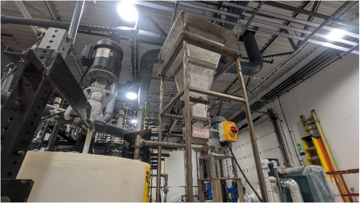
Figure 3 – RapidSX™ Automated Leaching Feeder
