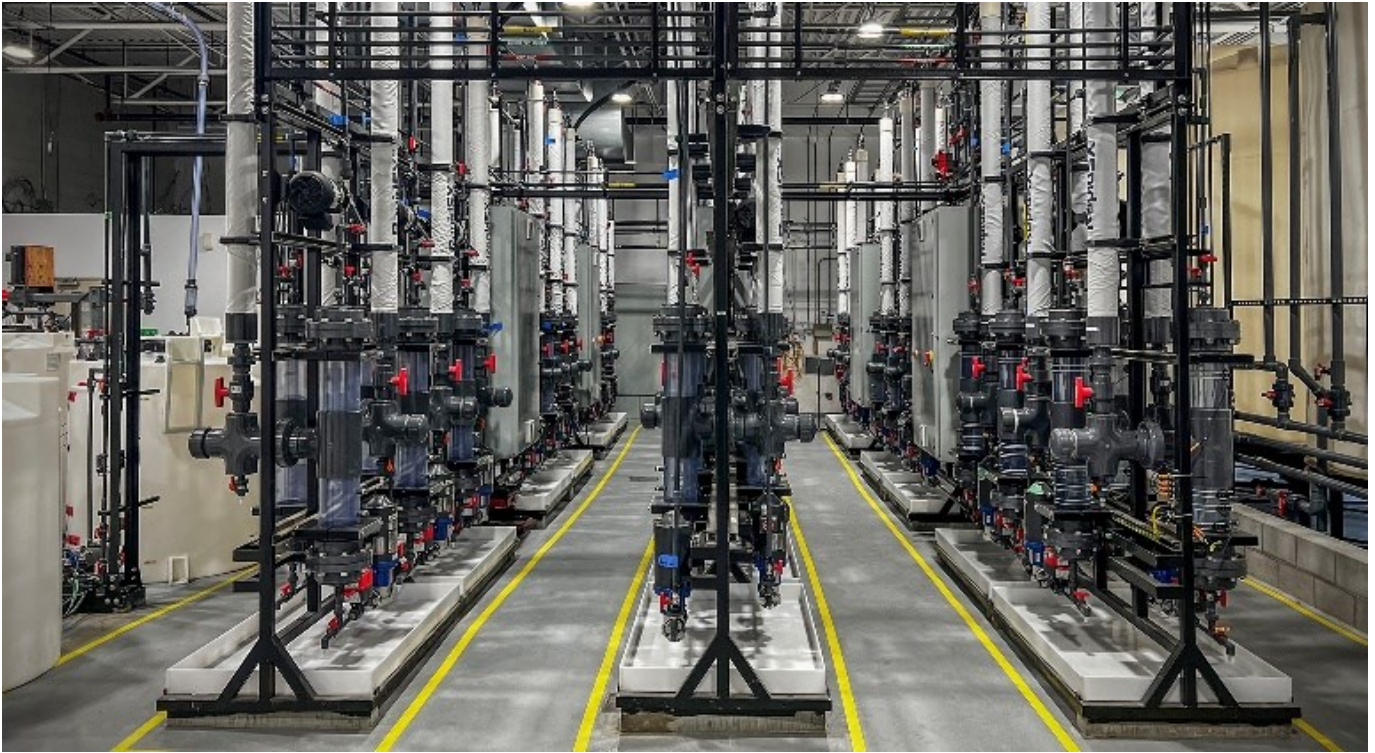
Figure 1 – 52-Stage RapidSX™ Demo Plant
