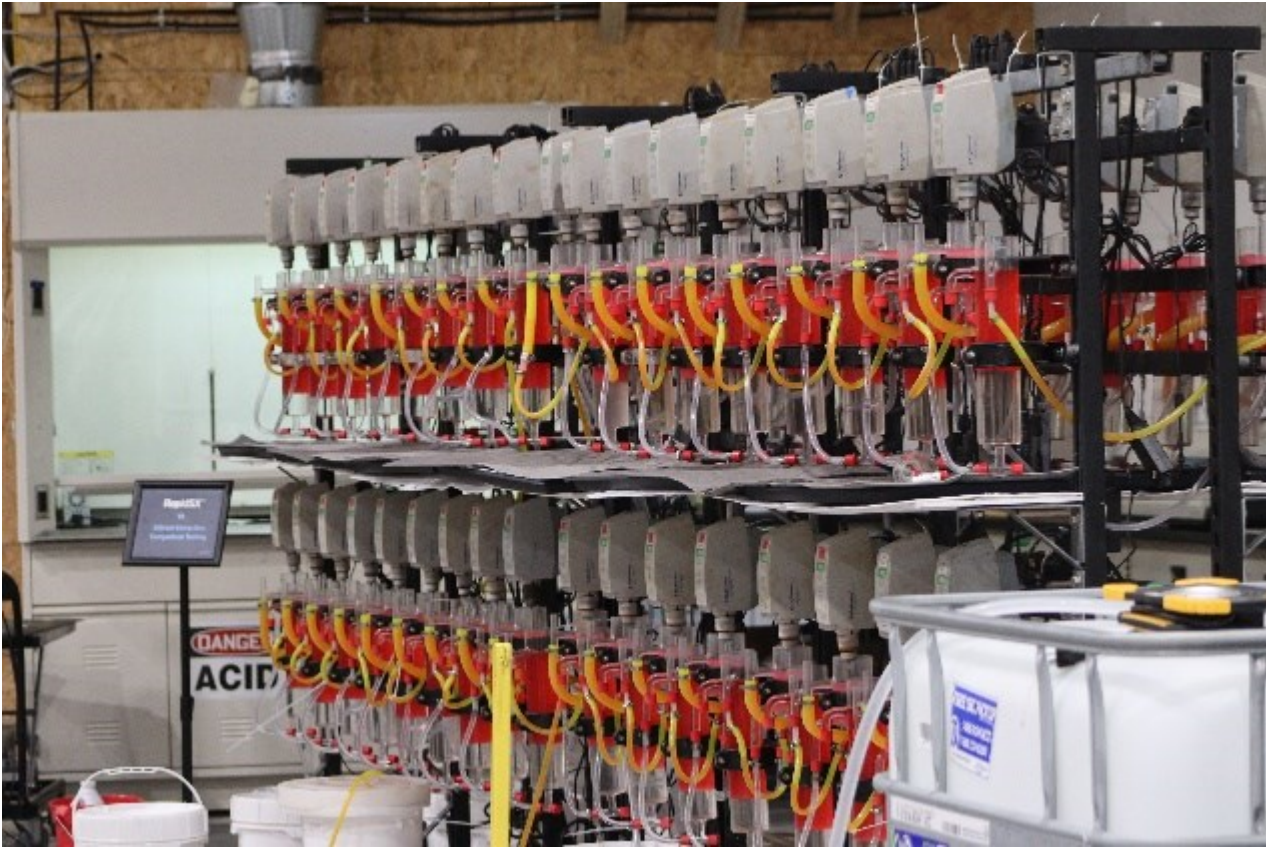
Figure 2 – 52-Stage CSX Pilot Plant
