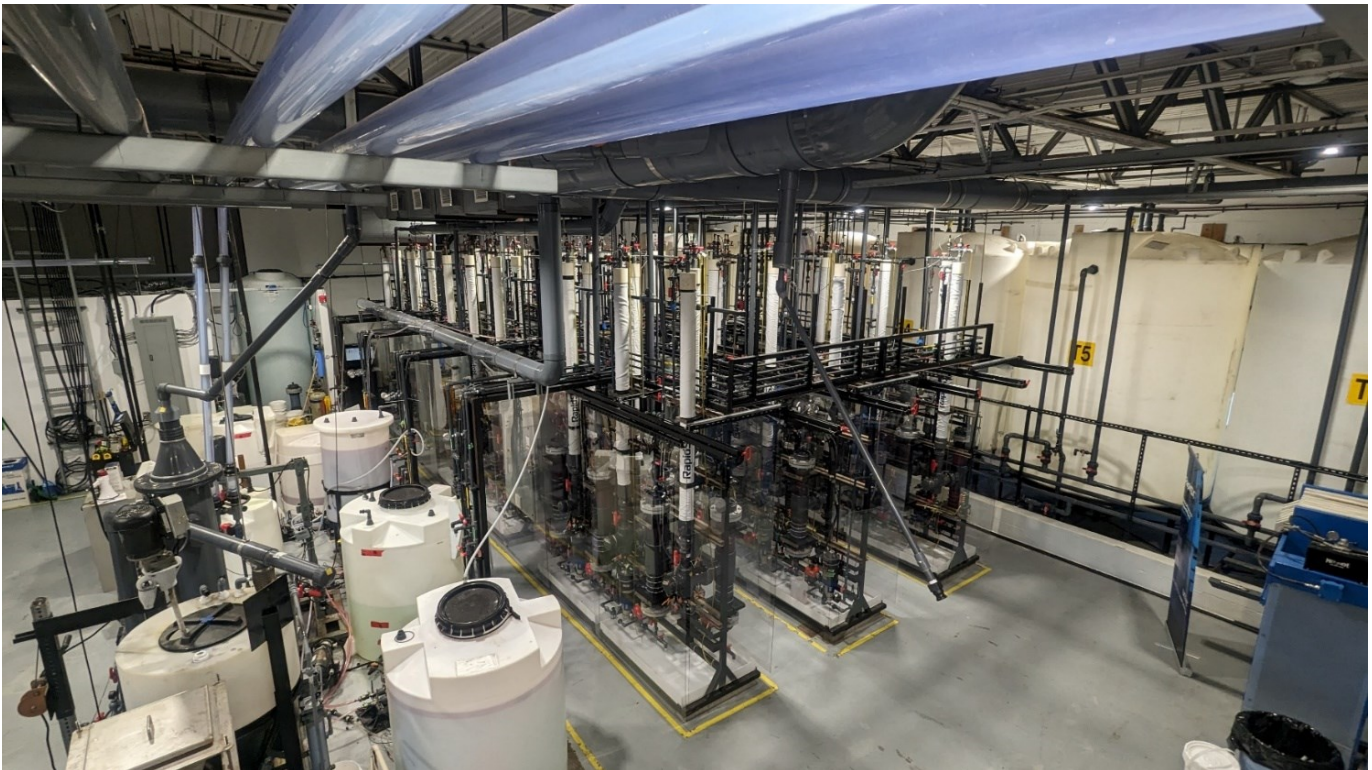
Figure 1 – Ucore's 52-stage RapidSX™ Commercial Demo Plant in Kingston, Ontario
