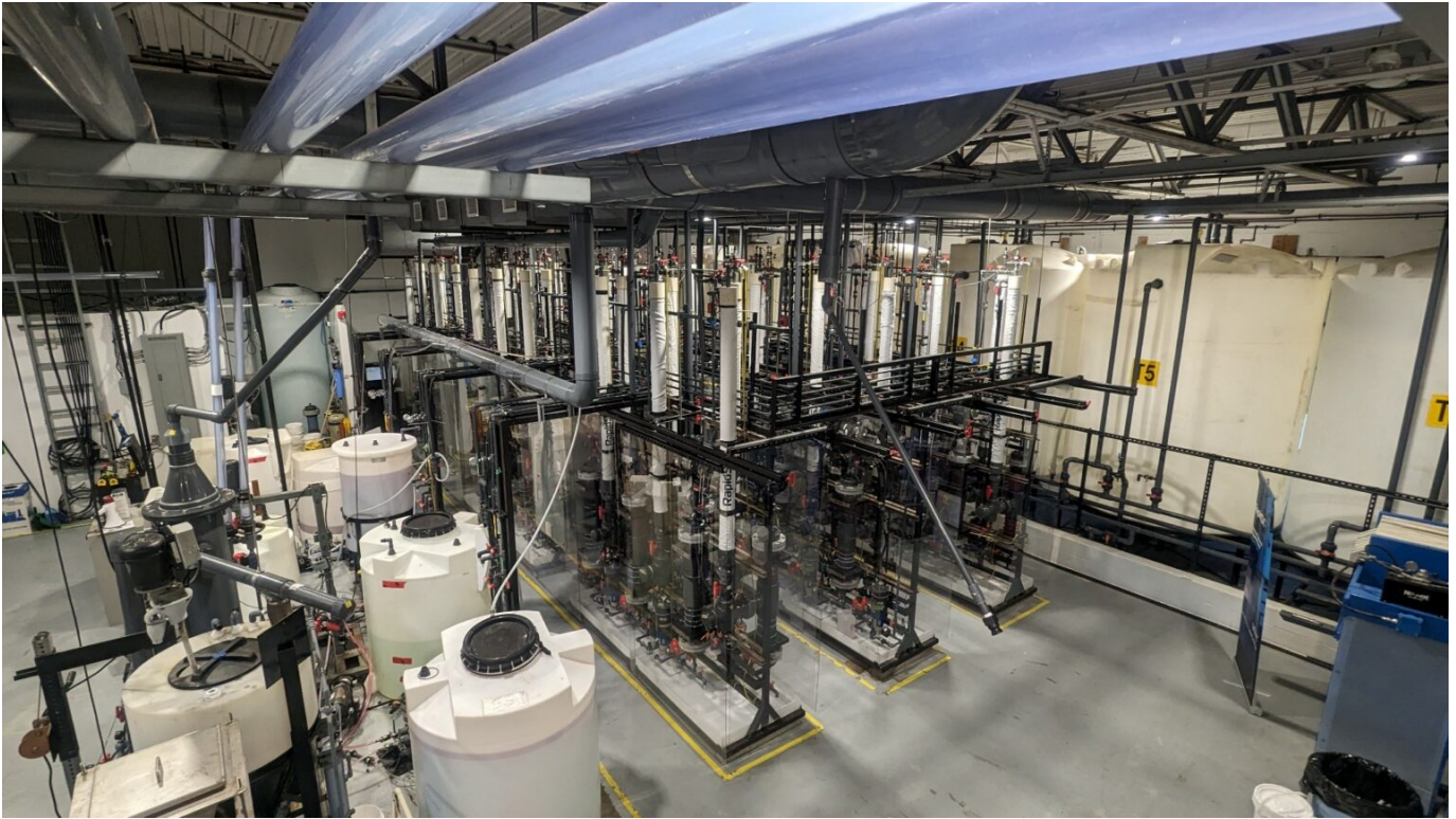
Figure 1 – The RapidSX™ Demo Plant Machine at the Kingston CDF
