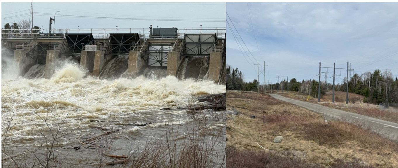
Figure 3. (a) Sturgeon Falls Power Dam and (b) Crystal Falls Power Lines on Property
